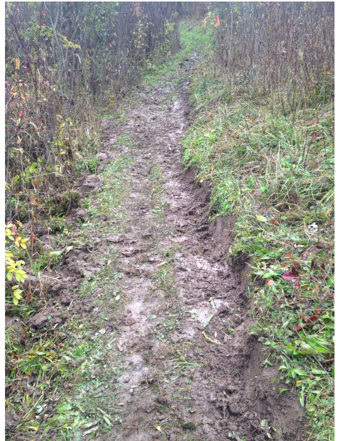
A section of the Seneca Trail at The Apple Farm that got some cut and fill by the Order of the Arrow scouts on Nov. 2, 2013. Photos by Rich Coloccia.
