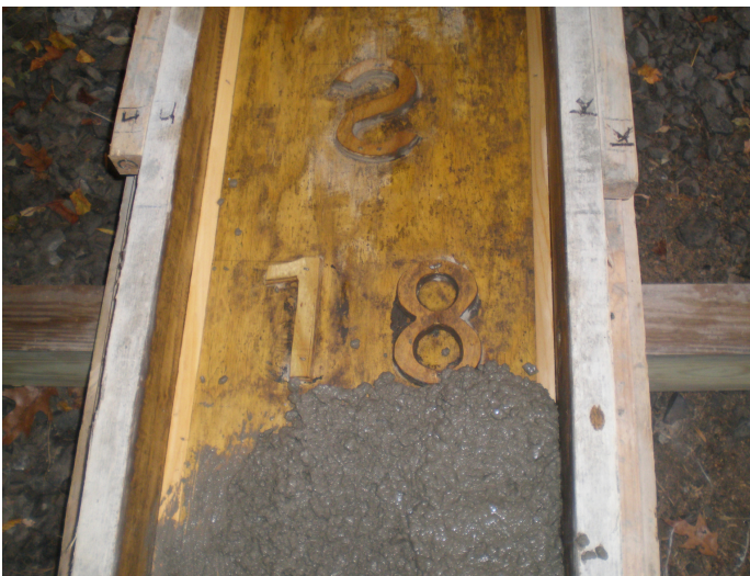
The form for mile marker 81. This one will be located on the Auburn Trail in Farmington.
